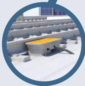
Cable for axle counters
